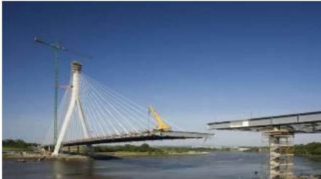
Suir Cable Stayed Bridge. 230 main Span (Waterford, Ireland). Fernandez Casado SL (completed in 2009).
